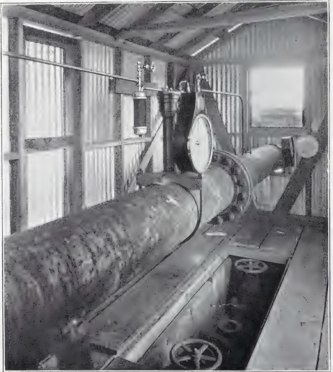
Fig. 11—ORIFICE METER ON LARGE GAS MAIN
